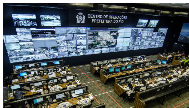
Figure 2. 80 meters screen with dashboard visualization at Centro de Operação Rio (COR). Source: (simi.org.br)
